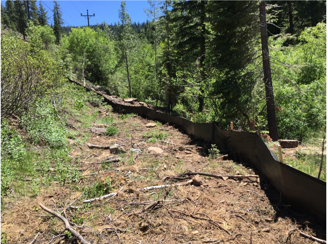
Photo 5: Silt fence installed along lower edge of ROW prior to construction activities (APM-SOILS-1).
